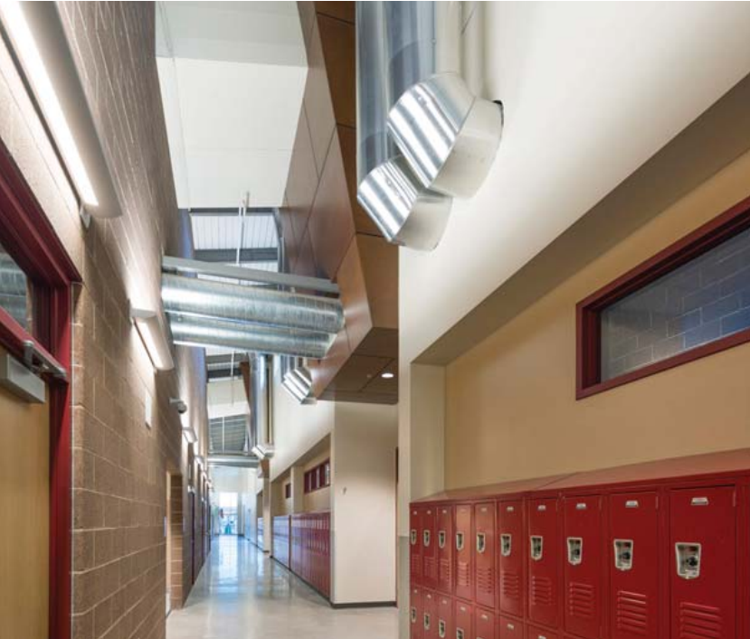
The exposed mechanical and electrical systems throughout the building are used as a teaching opportunity.
