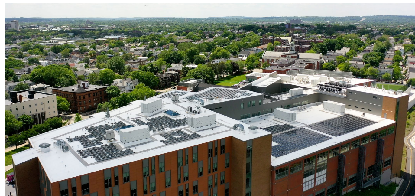
Solar PV Arrays
