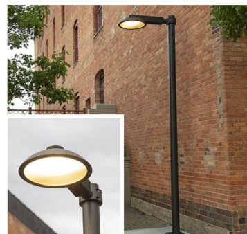
LED Pedestrian Light Post Manufactured by Landscape Forms 16' Post Height, Black Posts & Fixtures Location: Throughout Site
